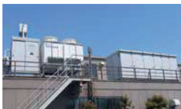
Gas Absorption Chiller
