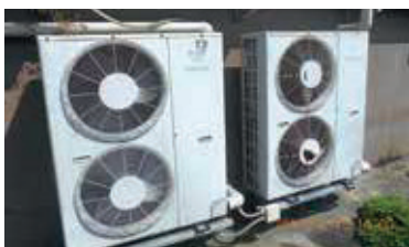
old split airconditioning system
